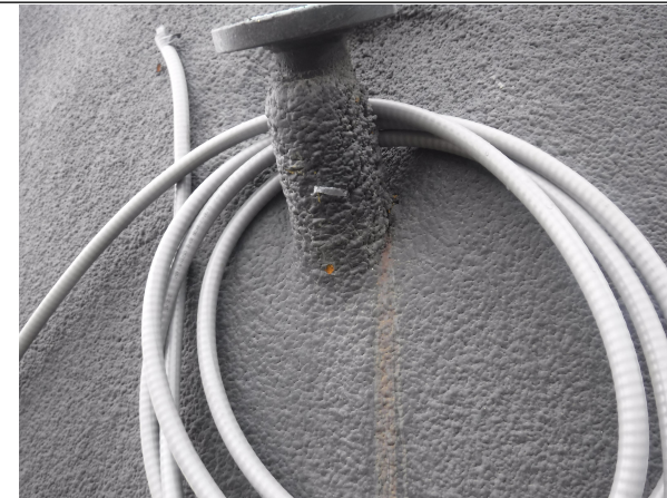
2" Scada nozzle rust rundown
