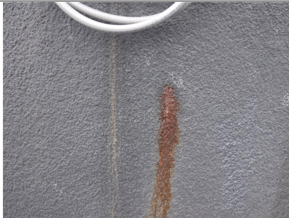
Rust rundown from insulation hole
