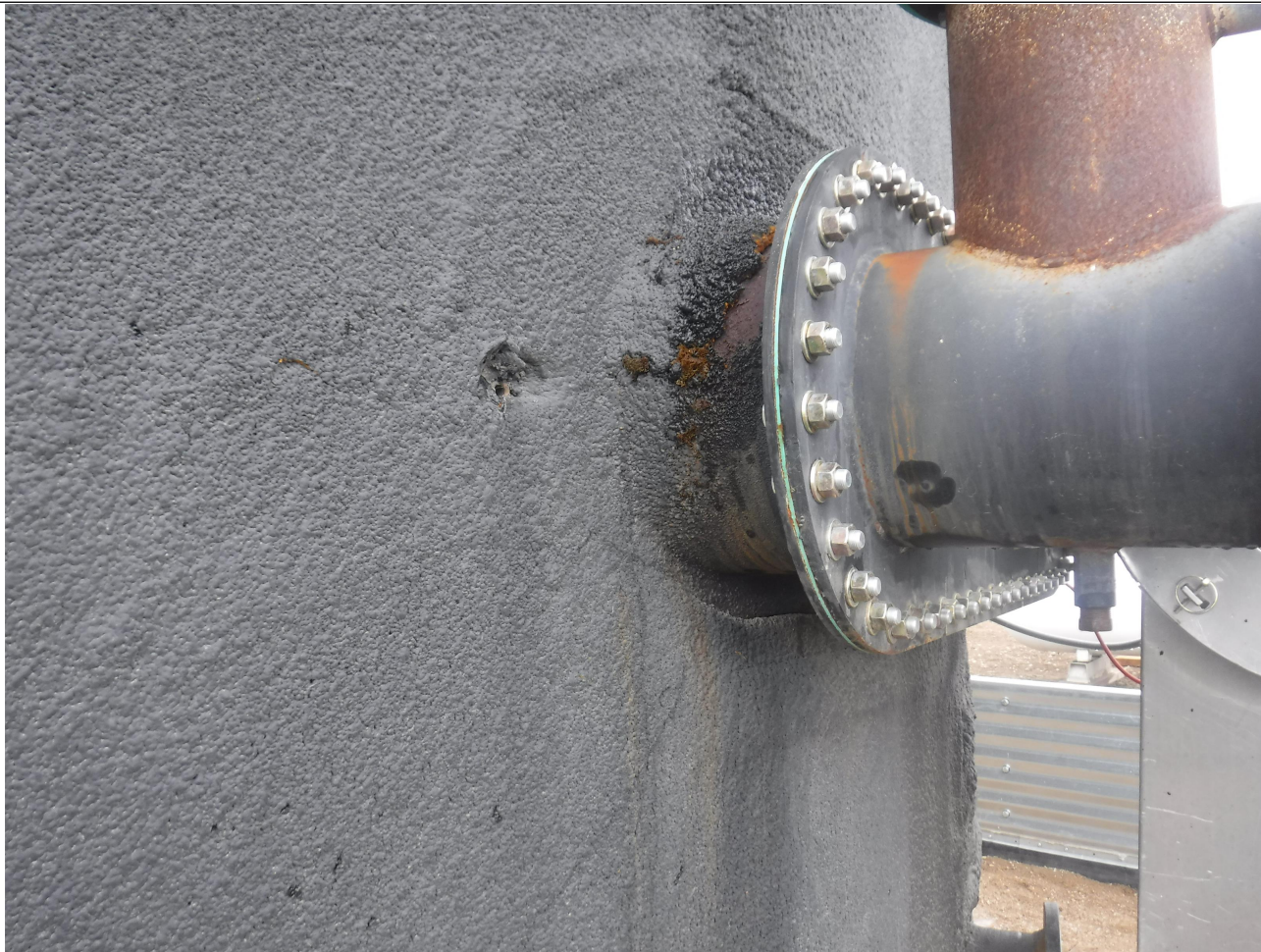
Rust/ Moisture rundown from firetube throat
