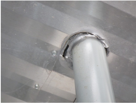
PIPING THROUGH ROOF SEAL FAILURE
