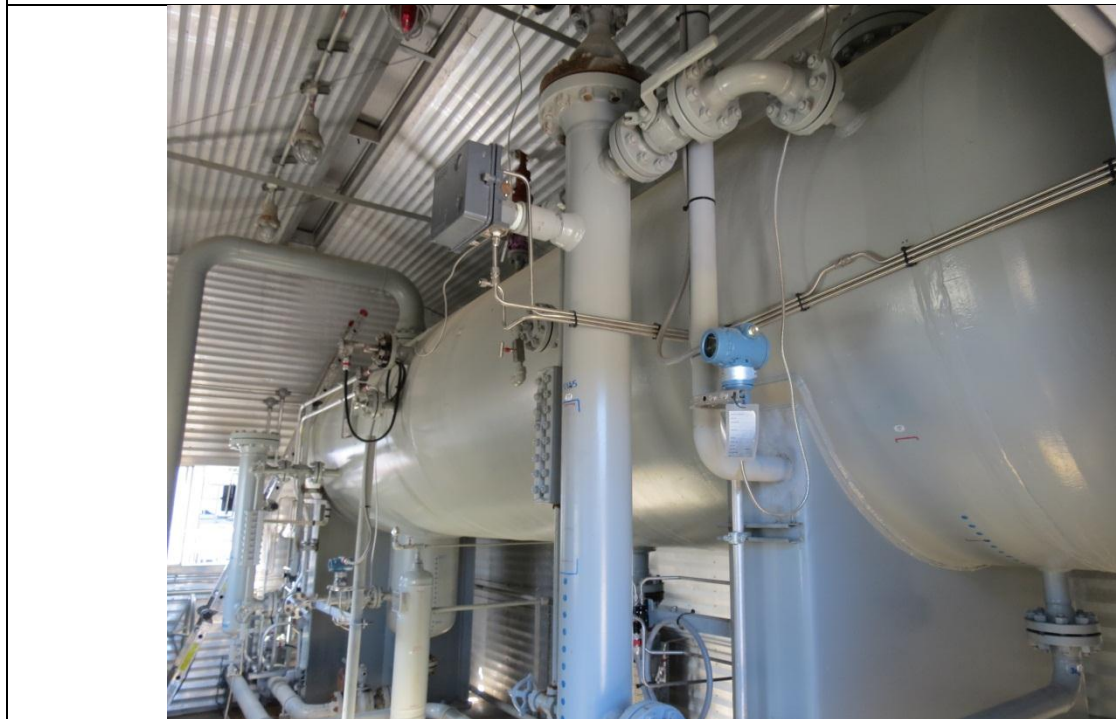
General View of the Vessel
