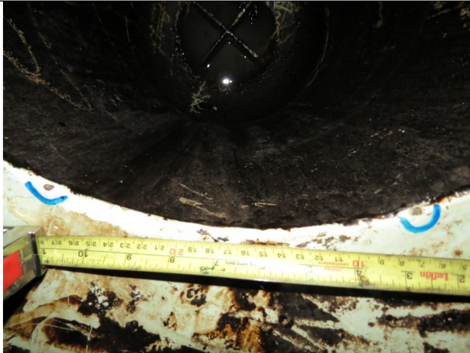
Small Coating Repairs Required Along the Drain Boot Weld
