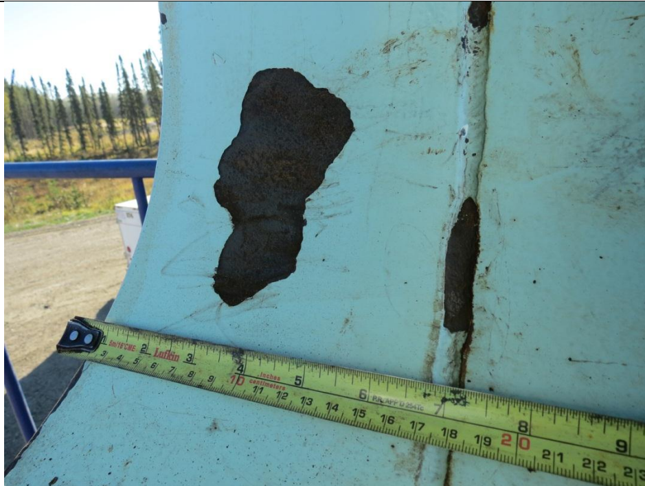
Coating Damage Inside Manway Nozzle
