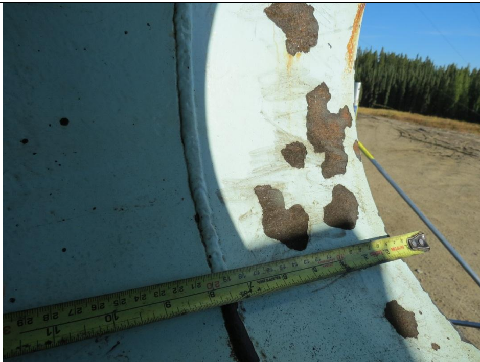
Coating Damage around Manway
