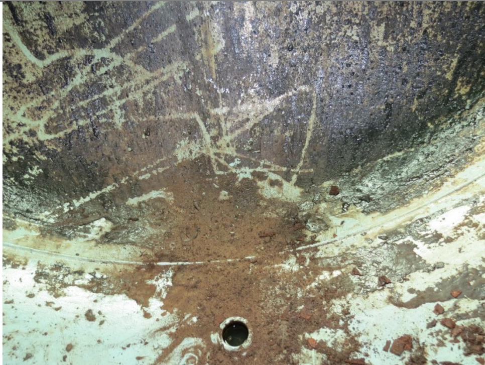
Debris along Bottom Shell
