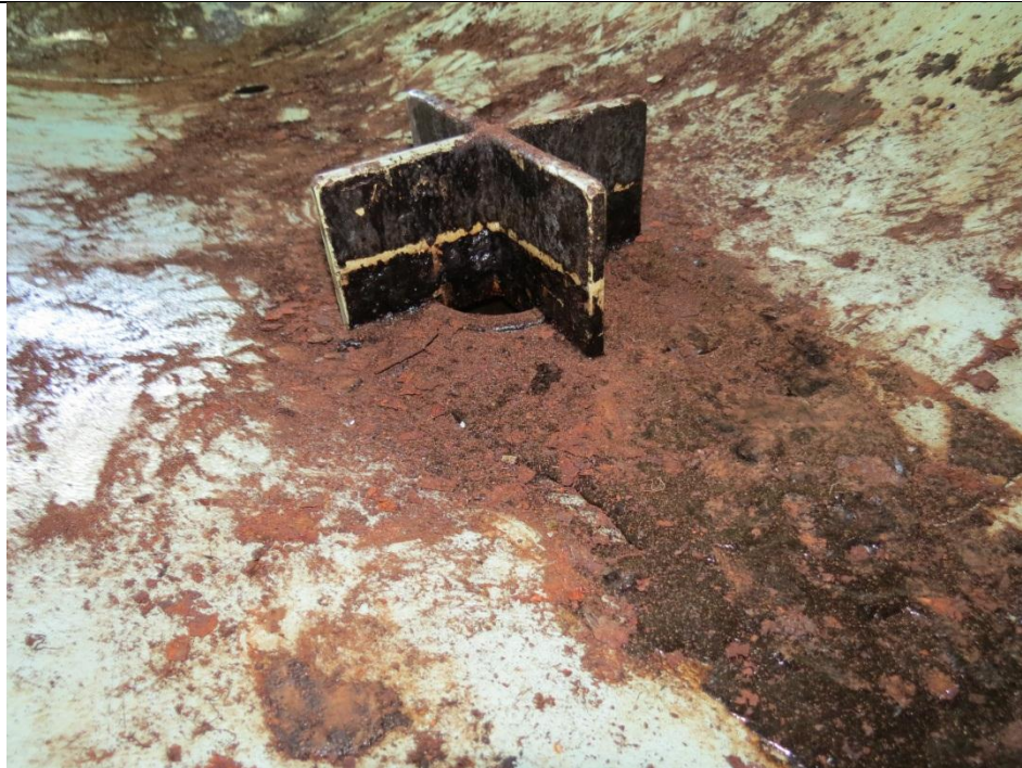
Vortex Breaker and Debris Deposits on Bottom Shell
