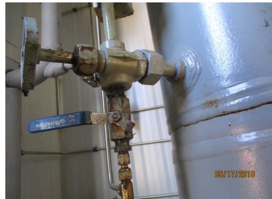
Lower Sight Glass Leak
