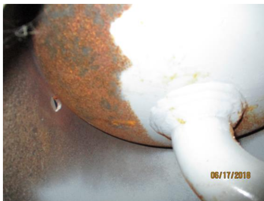
Surface rust on lower head and drain nozzle
