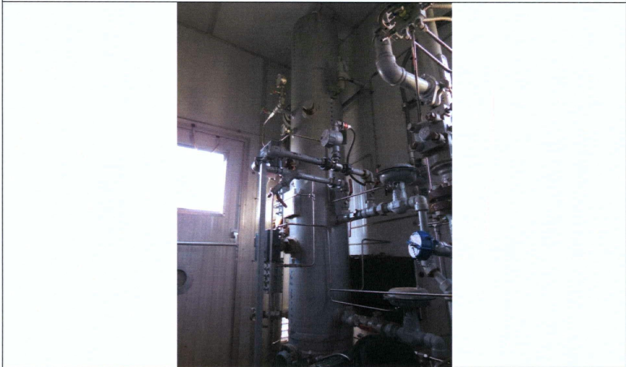
General View of the Vessel
