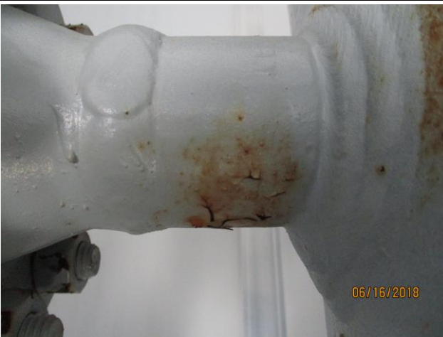
Coating failure on inlet nozzle
