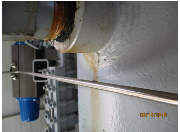
Leak noted on instrument connection
