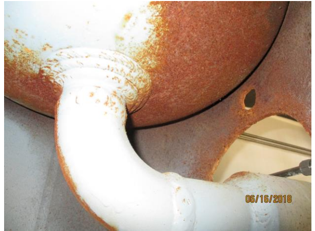
Surface rusting on lower head and drain
