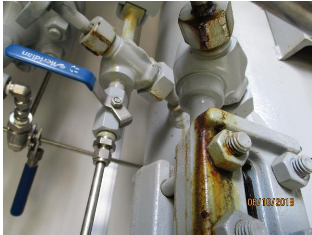
Leaking sight glass connection
