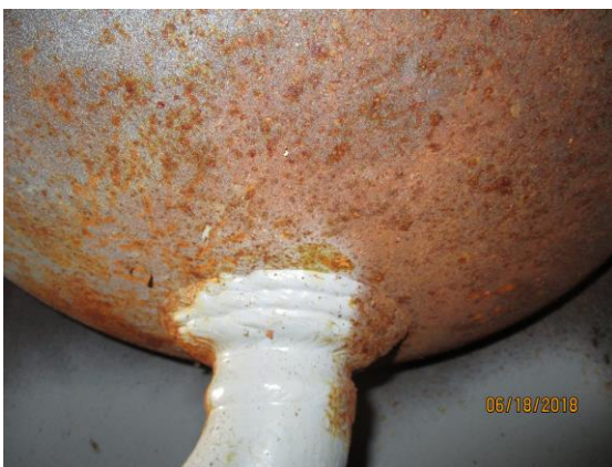
Lower head and Drain surface rust
