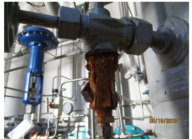
Lower sight glass leak
