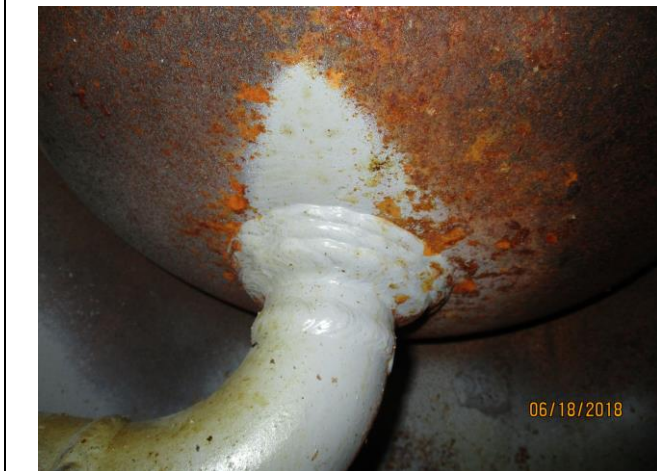
Lower head and Drain surface rust
