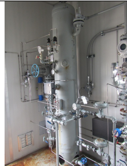
VESSEL AND PSV OVERVIEW
