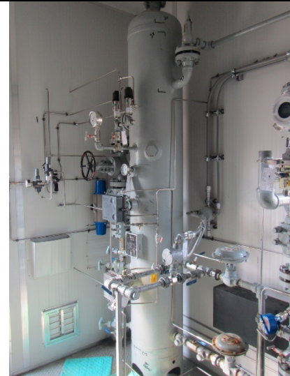
VESSEL AND PSV OVERVIEW - A LEAK CAN BE HEARD FROM PSV, SEEMS TO BE FROM INLET THREADED CONNECTION
