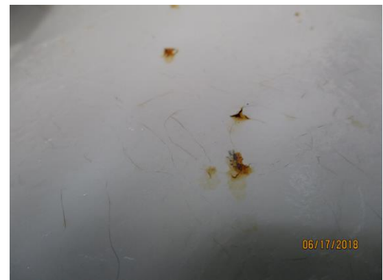
Coating failure on shell
