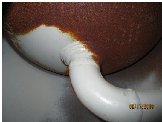
Surface rust on lower head and drain nozzle
