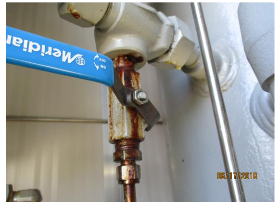
Lower Sight Glass Leak
