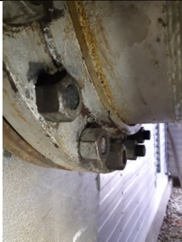
Short Bolting on Outlet Nozzle
