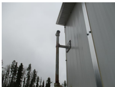
PSV DISCHARGE PIPING
