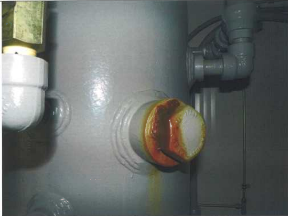
Leak stains from a 2" Plug on the Upper Shell
