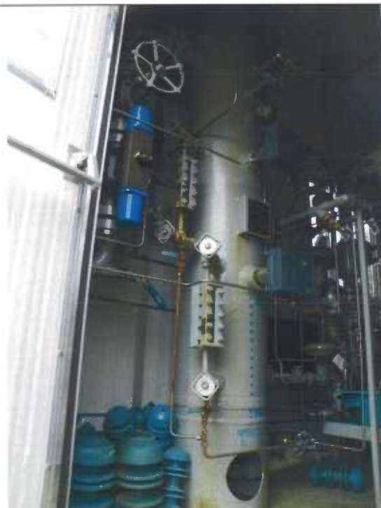
General View of the Vessel
