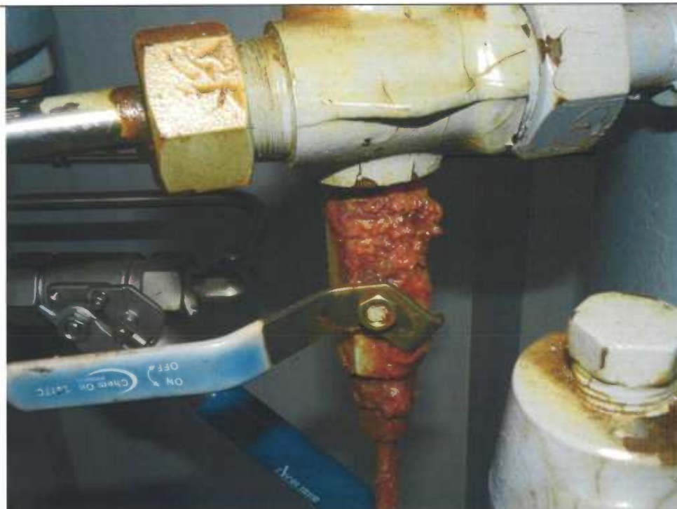
Signs of a Leak at the Bottom of the Sight Glass
