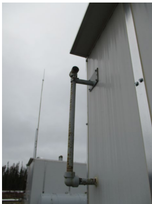
PSV DISCHARGE PIPING
