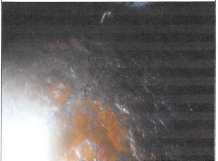
Typical of scale buildup on the floor
