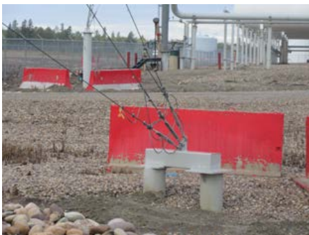
Guy Wire supports
