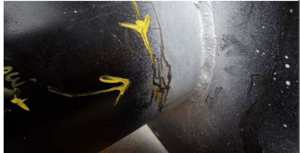
BURNER TUBE DEFECT SECTION
