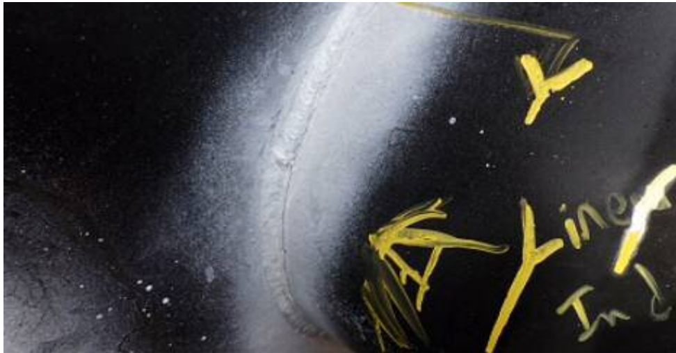
EXHAUST TUBE DEFECT SECTION
