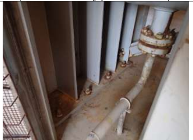
Support system at manway end
