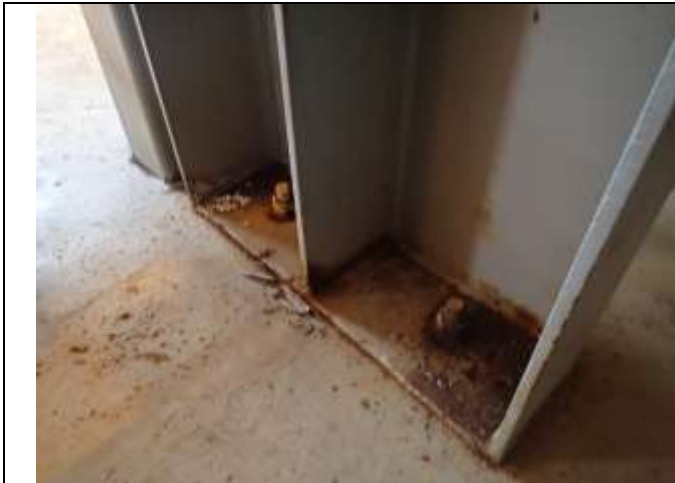
Support connection to skid. Rust flakes from paint failure/ minor external corrosion above.
