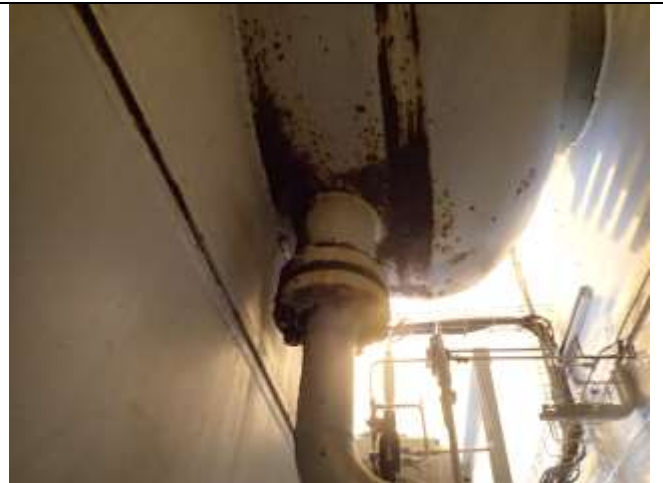
Paint failure area with minor external surface corrosion less than .005 in deep on east end. Not an integrity issue at the time of inspection.
