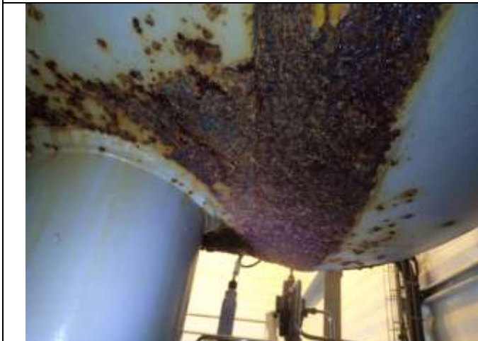
Close up of paint failure/external corrosion area.
