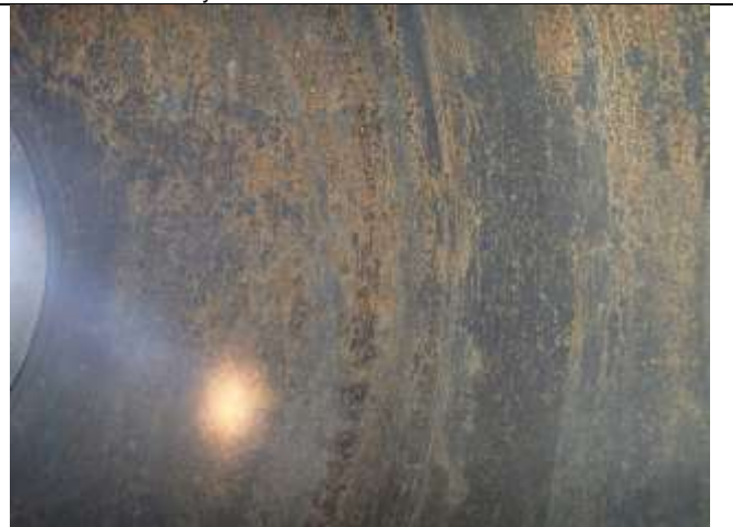
May 2017 Internal – Outlet end of shell. Typical all around with no relevant indications of corrosion/erosion or mechanical damage.
