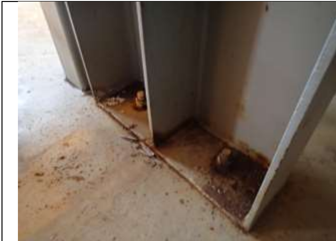
Support connection to skid. Rust flakes from paint failure/ minor external corrosion above.
