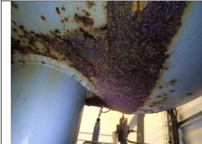
Close up of paint failure/external corrosion area.
