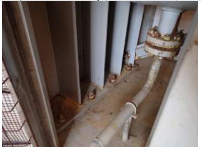
Support system at manway end
