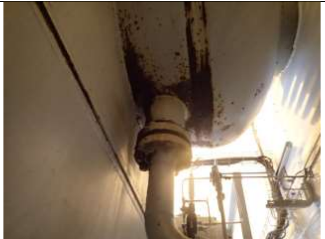
Paint failure area with minor external surface corrosion less than .005 in deep on east end. Not an integrity issue at the time of inspection.
