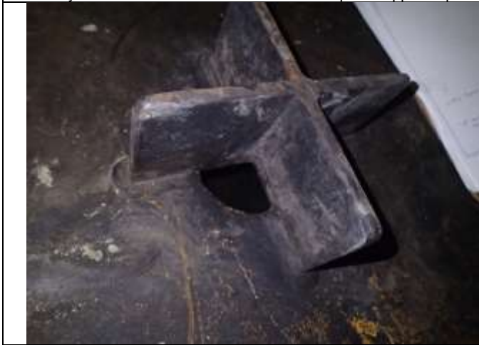
May 2017 Internal – Vortex breaker on water dump nozzle
