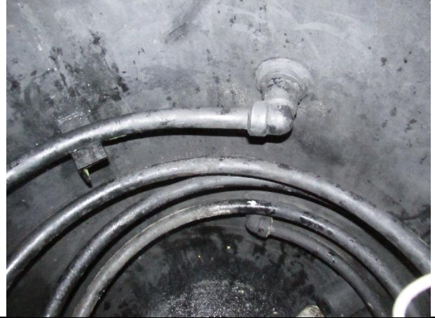
Internal coil attachment and supports
