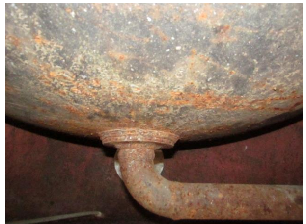
Bottom head general corrosion
