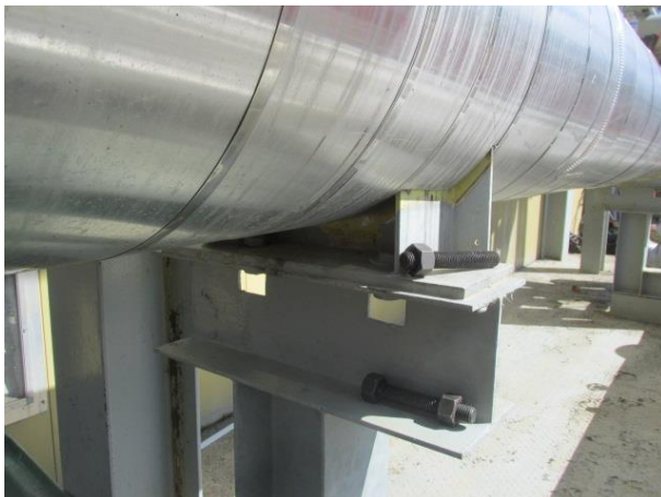
Saddle supports bolted to beams
