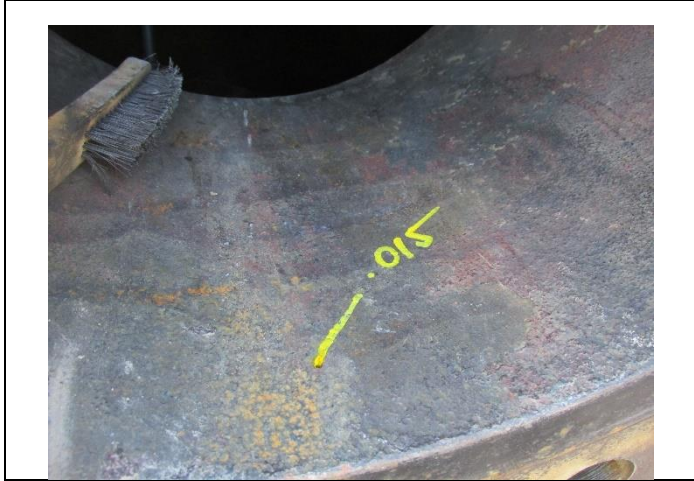
General corrosion on bottom of manway nozzle throat
