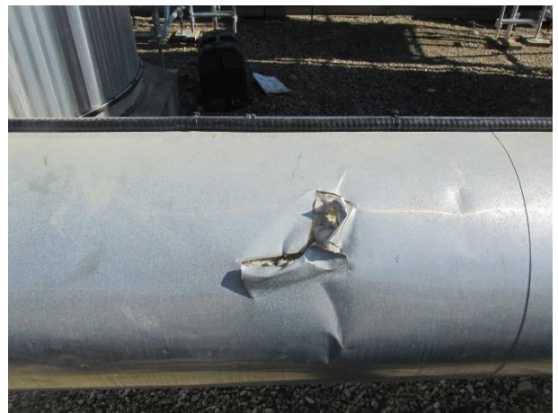
Bottom head piping cladding damage
