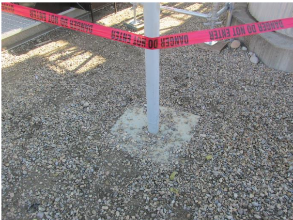
Temporary support for gas outlet piping, support post resting on ground
