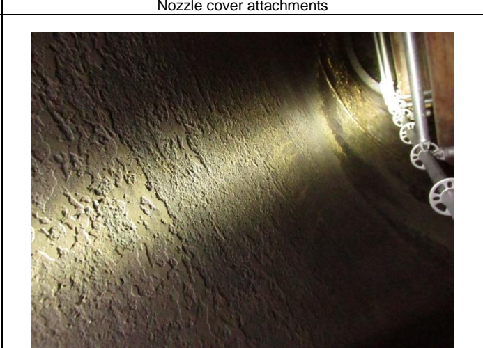
Bottom shell general corrosion
