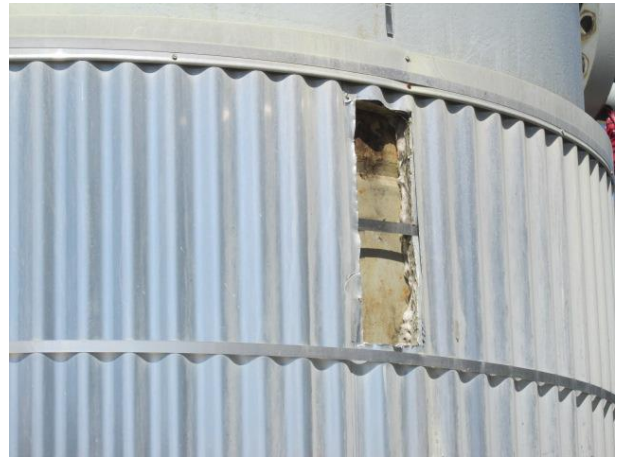
No coverplate on skirt cladding inspection cut out
