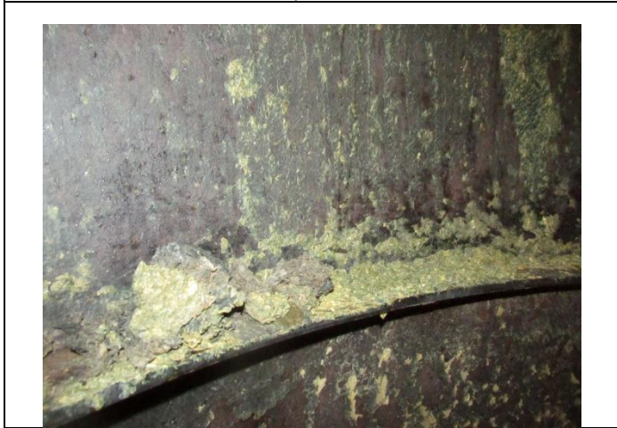
Top demister ring, no demister in use within vessel
