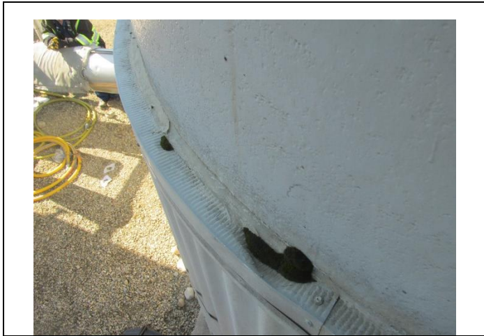
Moss growing at top of skirt cladding
