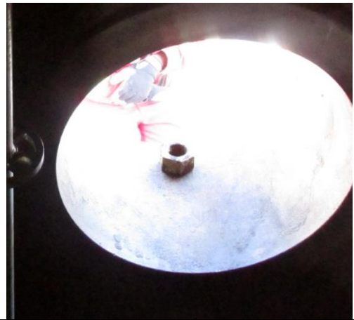
Loose bolt found on top of demister ring removed from vessel
