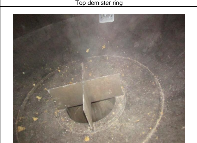
Bottom head and vortex breaker
