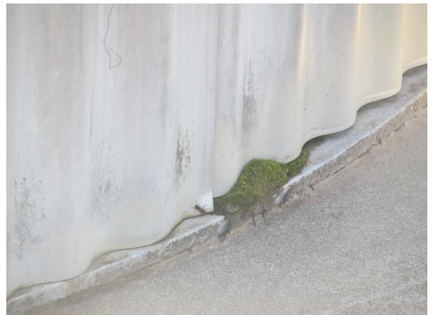
Moss growing at base of skirt cladding
