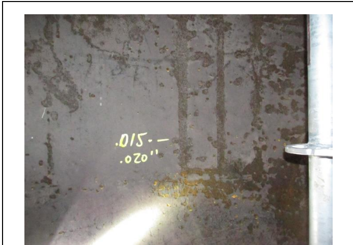
Bottom shell general corrosion
