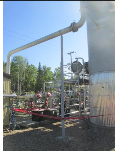
Temporary support for gas outlet piping, support post resting on ground
