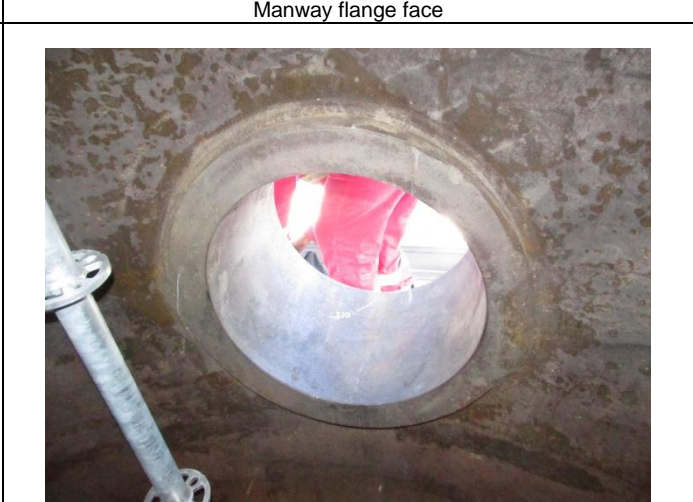
Manway and shell
