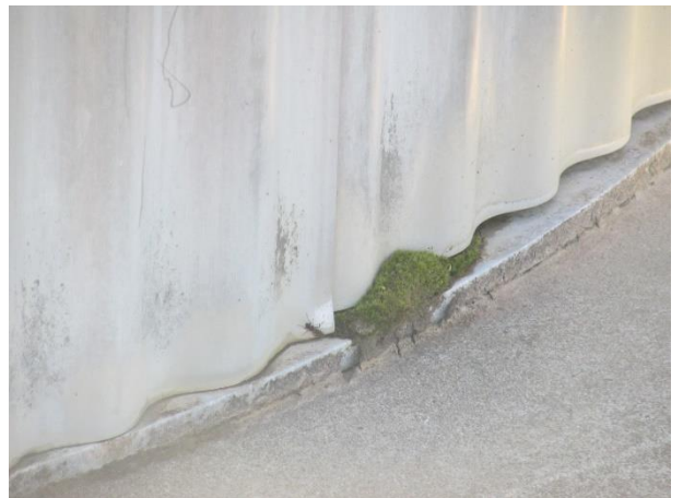
Moss growing at base of skirt cladding
