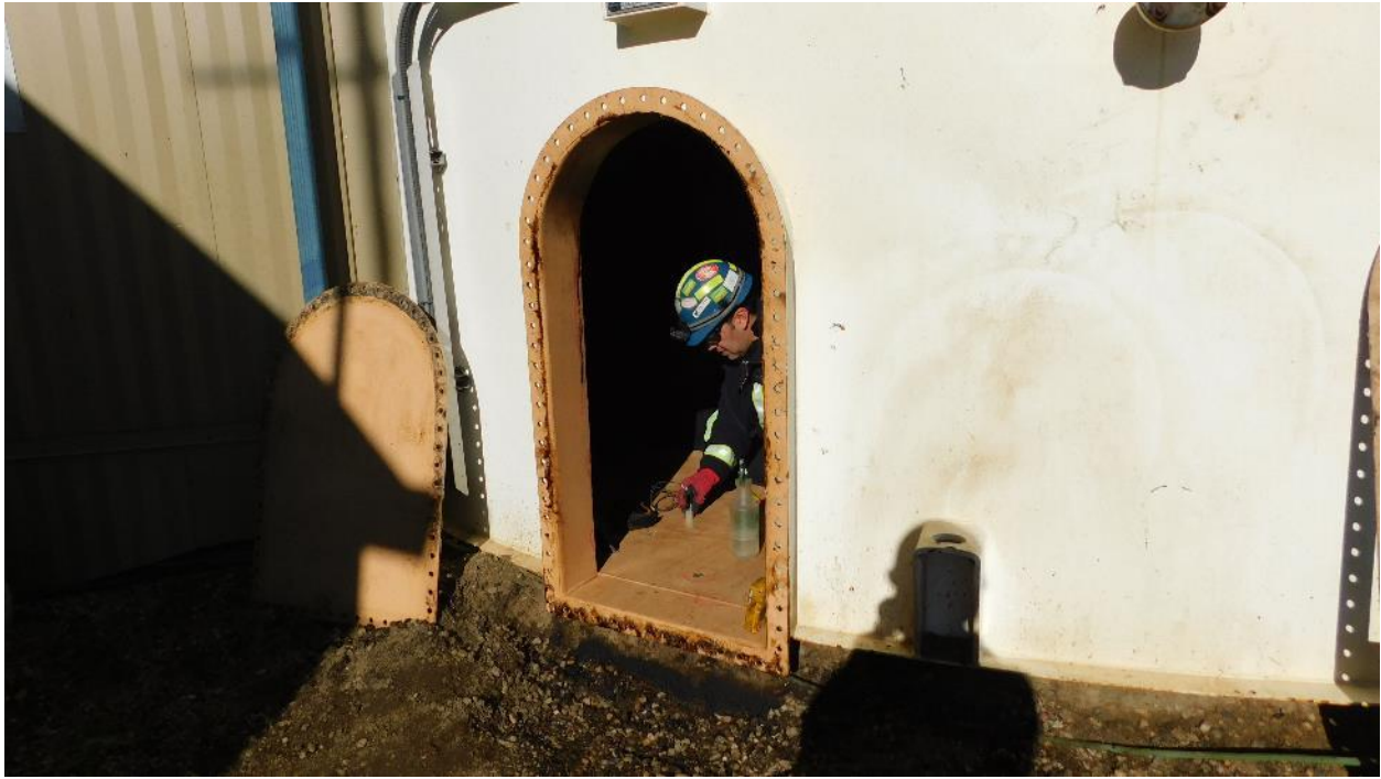
Photograph 17: Nameplate Entrance Manway
