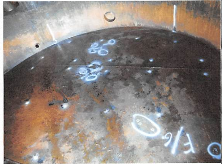
Areas of fill / grind sting gouge marks in floor
