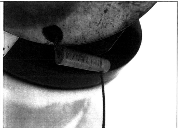
West block valve seal
