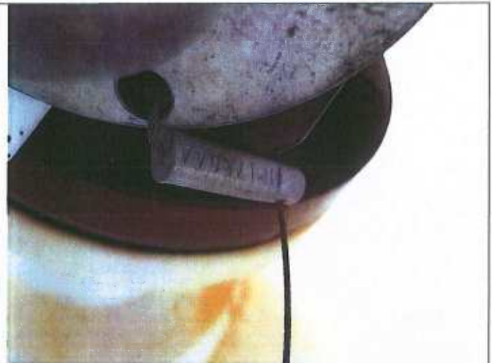
West block valve seal
