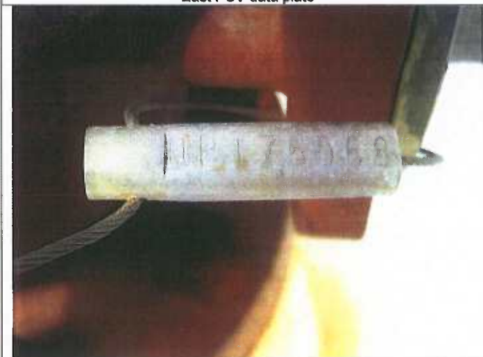
East block valve seal
