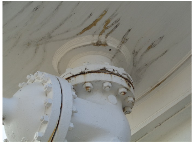
Flange paint deterioration
