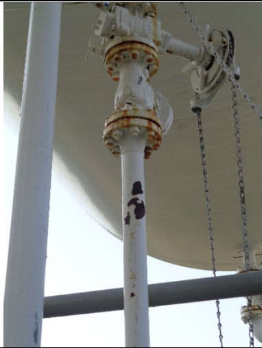
Piping paint deterioration
