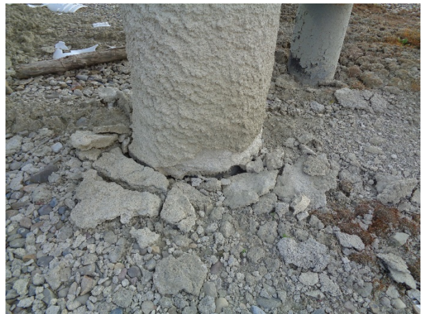
Minor damage to fireproofing at base of supports
