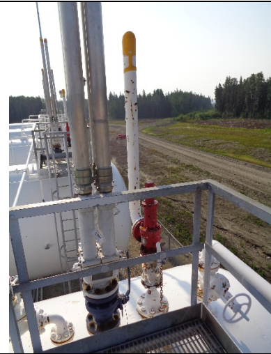
South PSV and North PSV manifold overview
