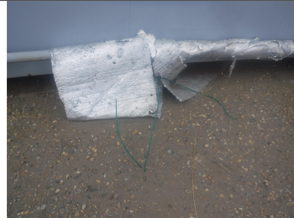
Cut ground wires
