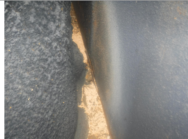
Debris build up between Containment and shell
