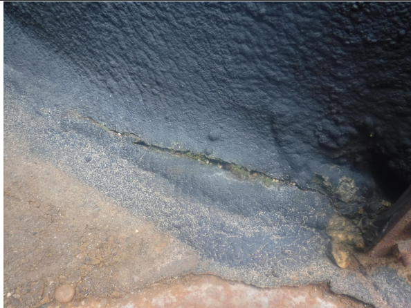
CUI suspecte at floor to shell
