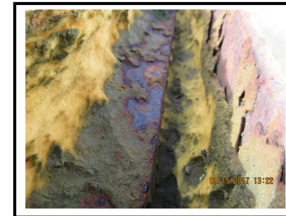
Insulation void exposing inner shell to environmental corrosion & deterioration.
