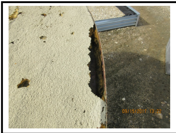
Insulation damage along roof edge.
