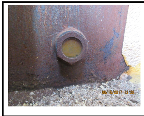
Interstitial space sight glass within heated enclosure. Obscured & requires cleaning.
